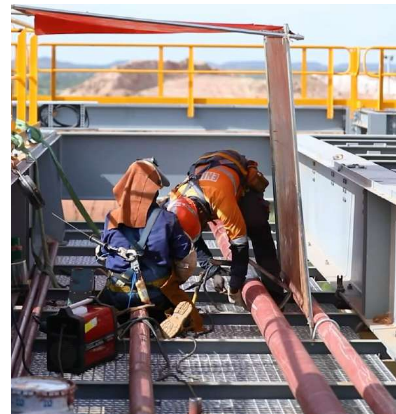
Welding work underway on site as part of the stage 1 hard rock expansion construction at the Bomboré Mine.
